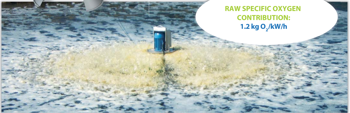
Flopulse 11kW in a leachate lagoon
